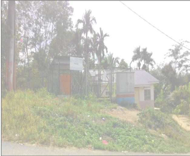
Photograph 5: Outdoor electric substation located in the Kg Orang Asli Ulu Kelaka managed by Tenaga Nasional Berhad (TNB)
